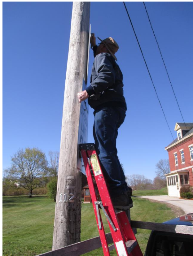
Handyman. Jim Noyes scales a telephone pole to remove a worn road sign in front of the Home for Aged Men in Newburyport.
